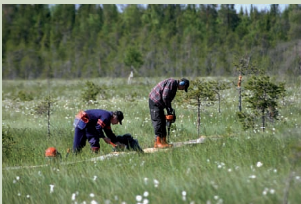
Building duckboards along a trail featuring traditional meadow culture in the Arctic Circle Hiking Area. Photo: Juha Paso.
