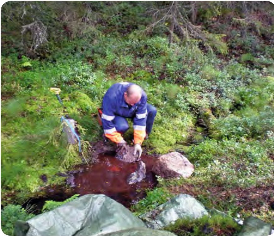
Figure 54. The water level in this spring was raised with the help of a small weir built about two metres away. Spring mosses were lifted out of the stream onto a tarpaulin for protection during restoration work. The water level eventually rose by about 5 cm. PHOTO: SARI KAARTINEN.
