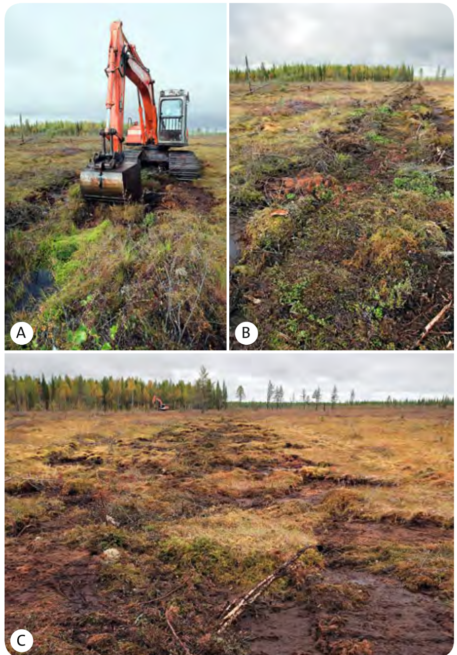
Figure 30. (A) The excavator driver filled in this ditch by driving up and down its entire length. On the outward journey he filled in the ditch compactly (B); and on the return journey he completed the peat embankments and channels for water (C). Trees had been felled in this naturally open peatland site during the previous winter. PHOTOS: PHILIPPE FAYT.
