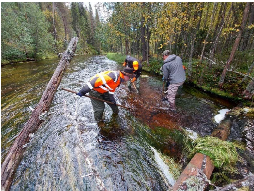
Figure 18. Restoration with Hartijoki method in Pirinoja, wooden deflector above the restoration area. Photo: Pirkko-Liisa Luhta.
