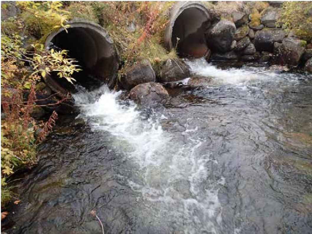
Figure 194. Culvert pipes under a private road in Vuohččojohka may prevent salmon parr ascending into the river. Photo: Aune Veersalu.
