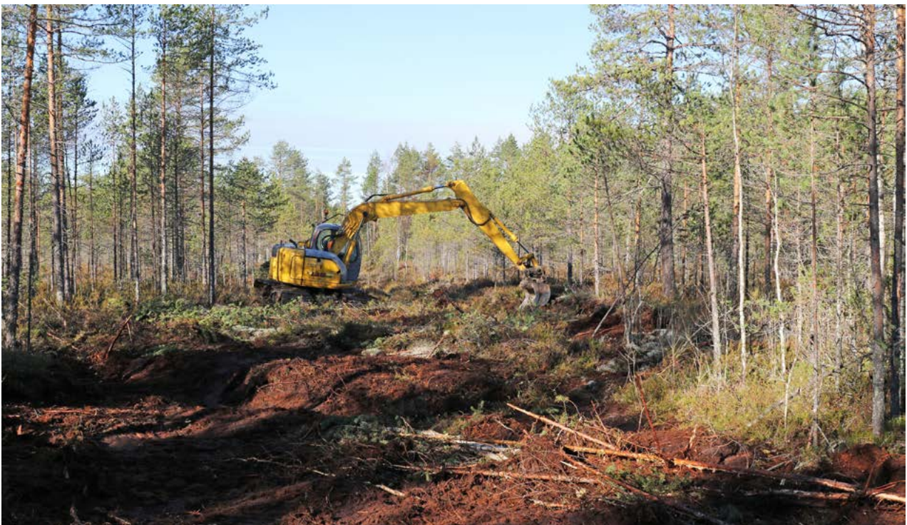
Bog woodland under restoration with ditches filled with an excavator. Photo: Maarit Similä.
