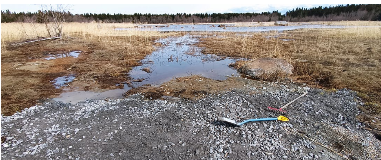
Figures 15 and 16. In Långviken, the goal of the restoration was to close two man-made channels and to restore the natural inlet and sill. Aggregate, clay and gravel for the work were found in situ and also obtained off-site. Photos: Ralf Wistbacka.
