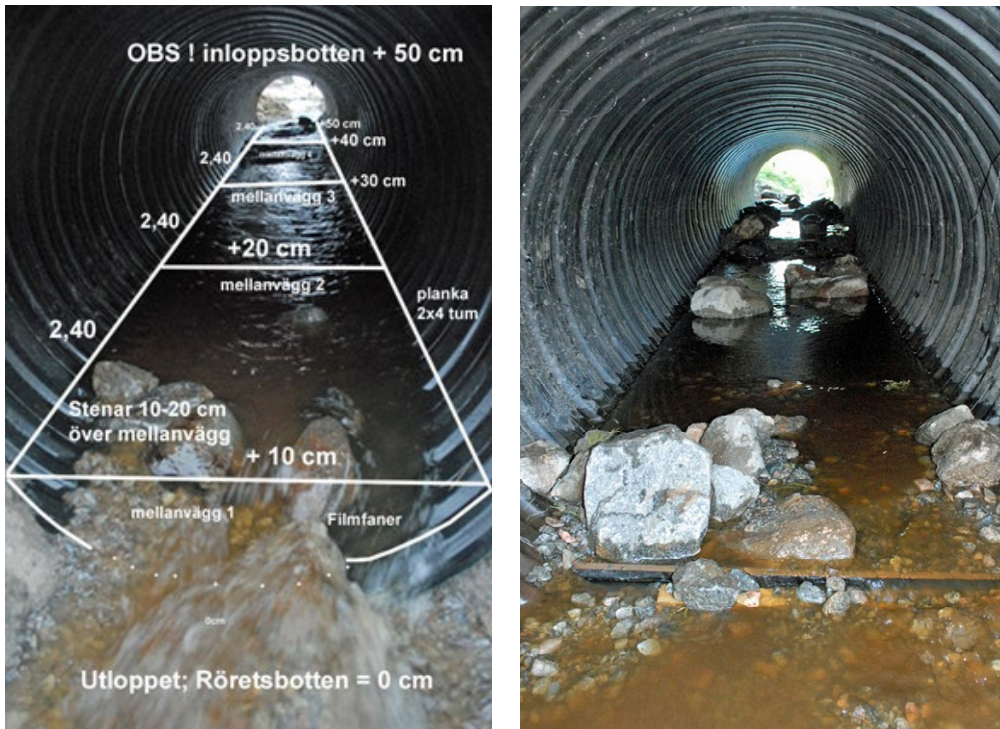
Figures 20 and 21. The channel to be restored had a steep slope, so a decision was made to build a fish pass inside the culvert and fill it with gravel and rocks, creating a natural, gradual slope where spawning fish can rest and pick up speed. The water level is still relatively low in this photo. Photos: Ralf Wistbacka 2013.
