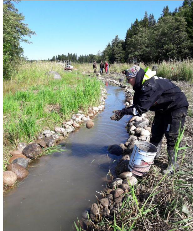
Figure 37. Plenty of stones are placed in the channel. Photo: Sanna Kuningas/Natural Resources Institute Finland.
