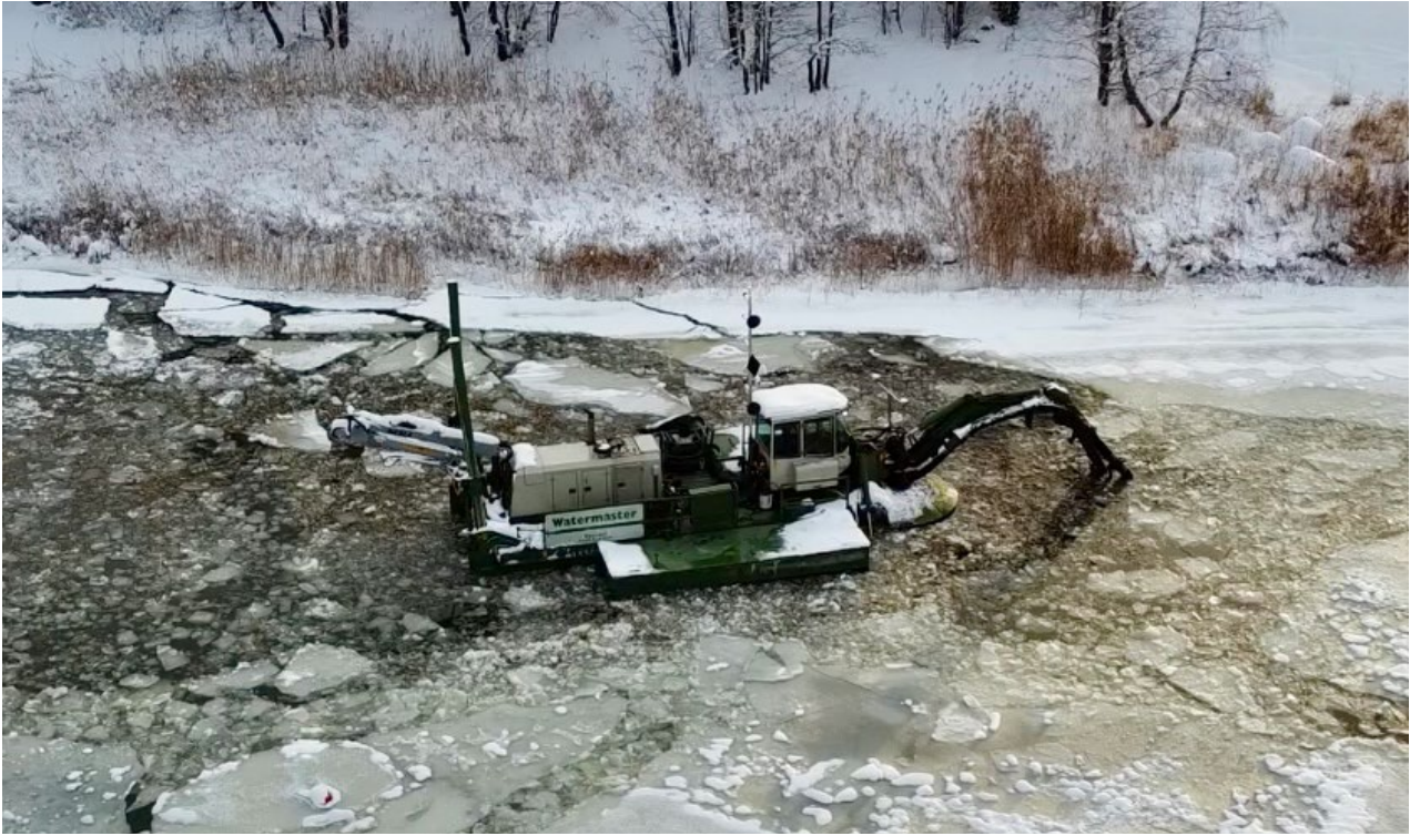
Figure 10. Suction dredging of the sediment in the straits of the Pappilansaari Islands, Hamina. Photo: Harri Huuho/MeriHamina Association.
